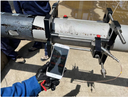
Fig. 1: Clamp on installation on high pressure hydrogen line
