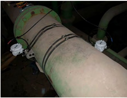
Picture 3. 50-year-old corroded pipe
