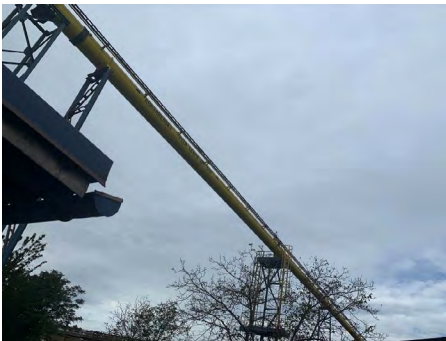
Picture 12. DN800 coke oven gas
