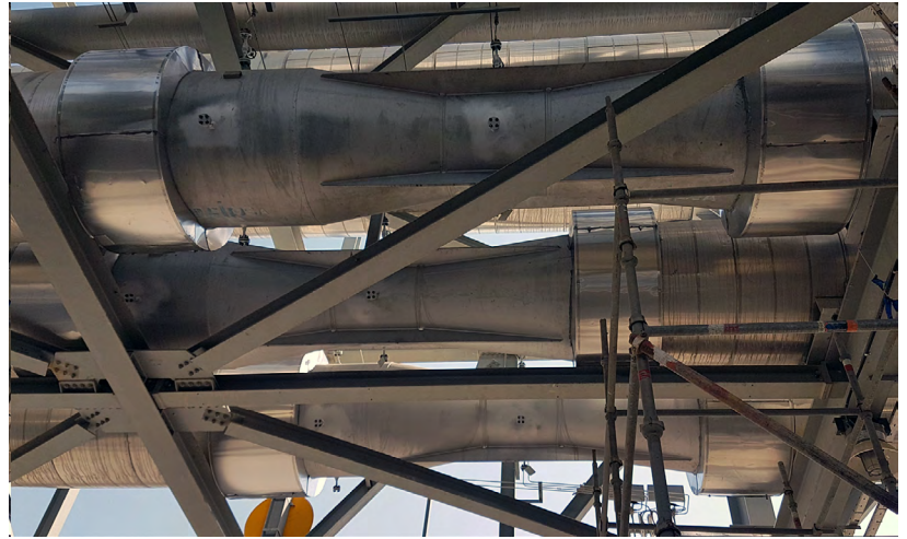
Figure 2: Former Venturi Flow meter
