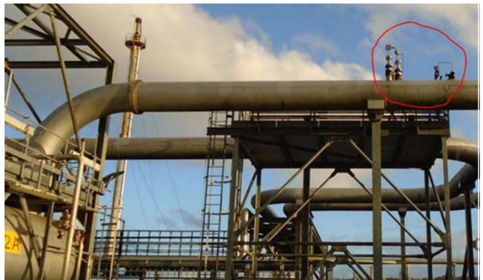
Fig 1. A 30" horizontal pipe 12 meters (39'+) above ground level
