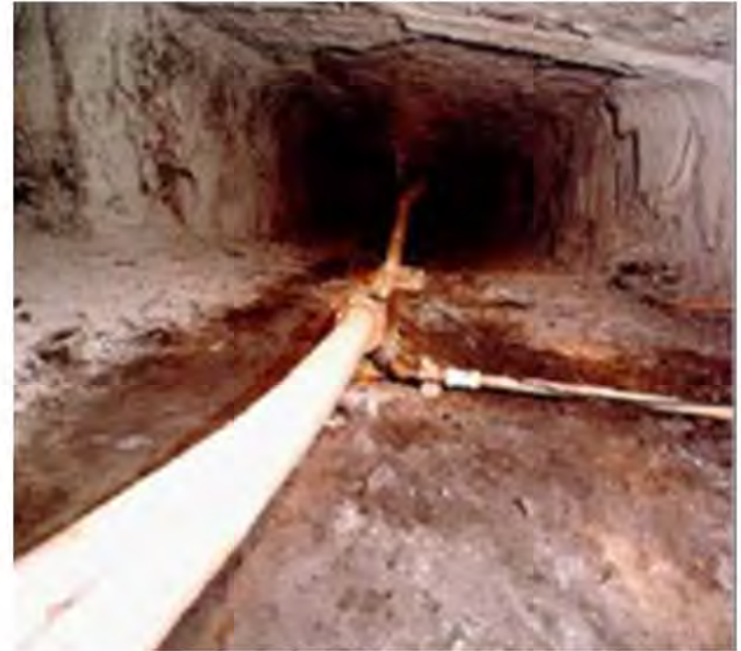
HDPE Gas Collection Piping
