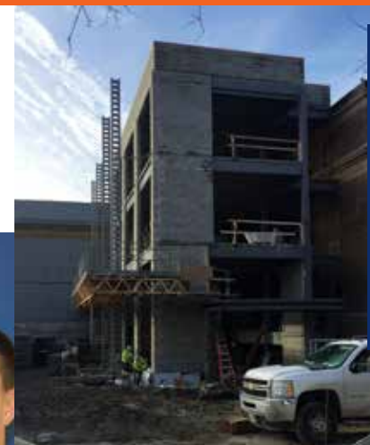
Annex for an Annex: An expansion on the southeast side of Chemistry Annex is part of a roughly $25 million renovation of the building, built in 1930. The work is scheduled to be complete this year.
