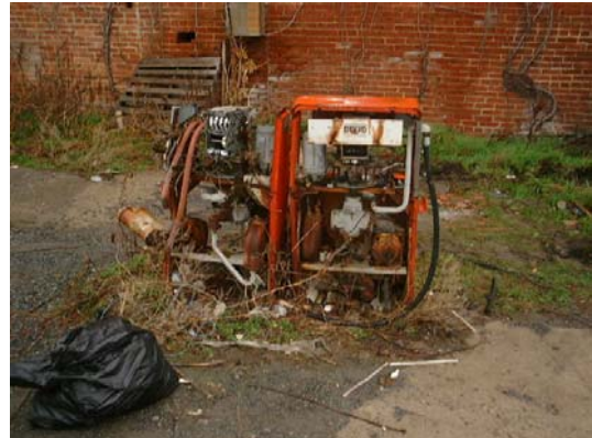
Fuel Dispenser in UST Area
