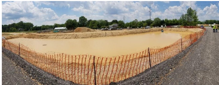
Figure 1 - Stormwater BMP with Turbid Waters
