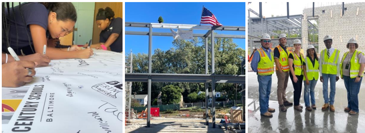
Photos courtesy of 21 st Century School Buildings Program; Banner Signing at Cross Country Elementary/Middle
