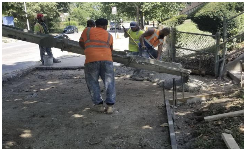
Sidewalk repairs by J. Villa Construction Co. on Braddish Avenue next to Katherine Johnson Global Academy. Photo by Mike Camper (Department of Transportation), August 9, 2022.
