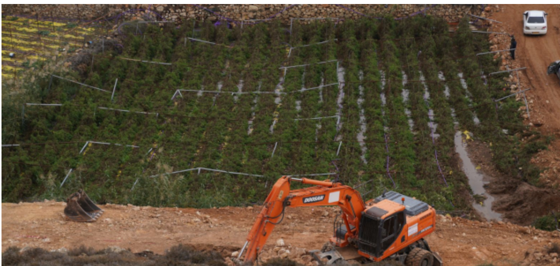
Construction of wetlands at each of the 3 farms in Al-Salt, Jordan and another 3 in Sa'ir, Palestine, to provide tertiary treatment to wastewater from the Wadi Shuayb Wastewater Treatment Plant in Jordan and the Wadi Al-Arroub Plant in Palestine.
