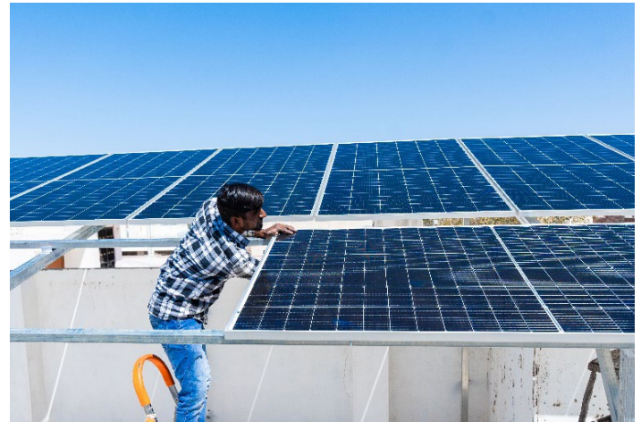
Indian worker installing solar panels on roof of house. Maintenance of photovoltaic panel system. Photo Credit: Adobe Stock - By Gajendra
