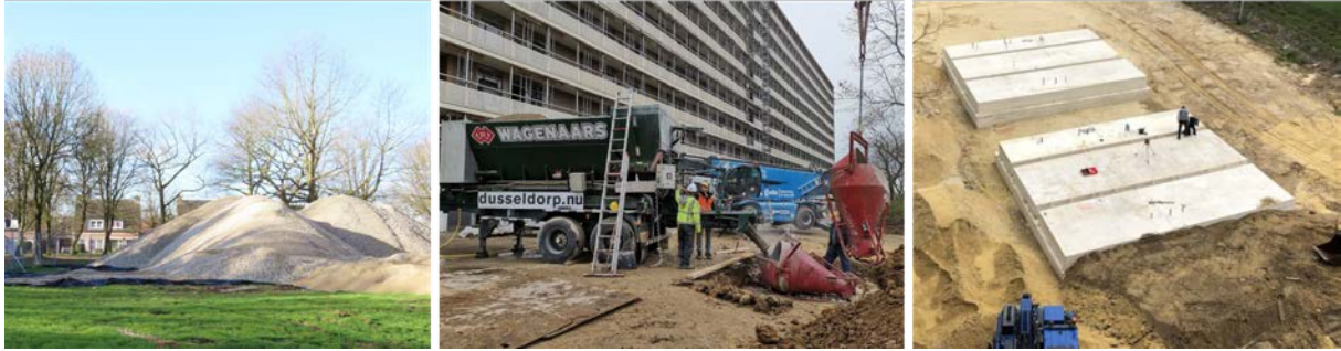
Figure 5: Aggregate for the foundation of three super circular estate houses has been reused from a donor building in the neighbourhood which has been demolished using conventional demolition techniques. Foundation of houses type A, B and C has been made with 100% reused aggregate.
