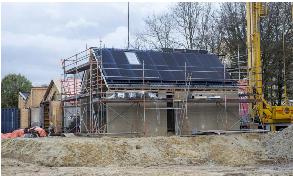
Figure 1: Construction of three UIA SCE houses in the row, first Type C, Type B and Type A
