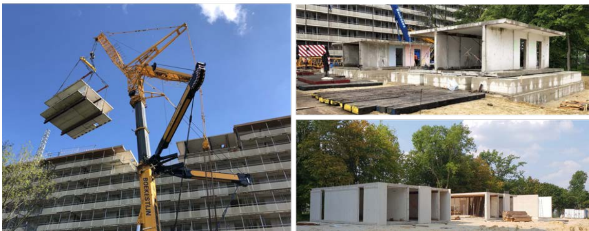
Figure 3: Recovery of 3D reinforced concrete units from outdated high-rise social housing building built in 60's and placement of 3D units on the foundation of super circular estate houses type A and type B
