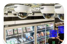
Enhanced Surveillance Systems
