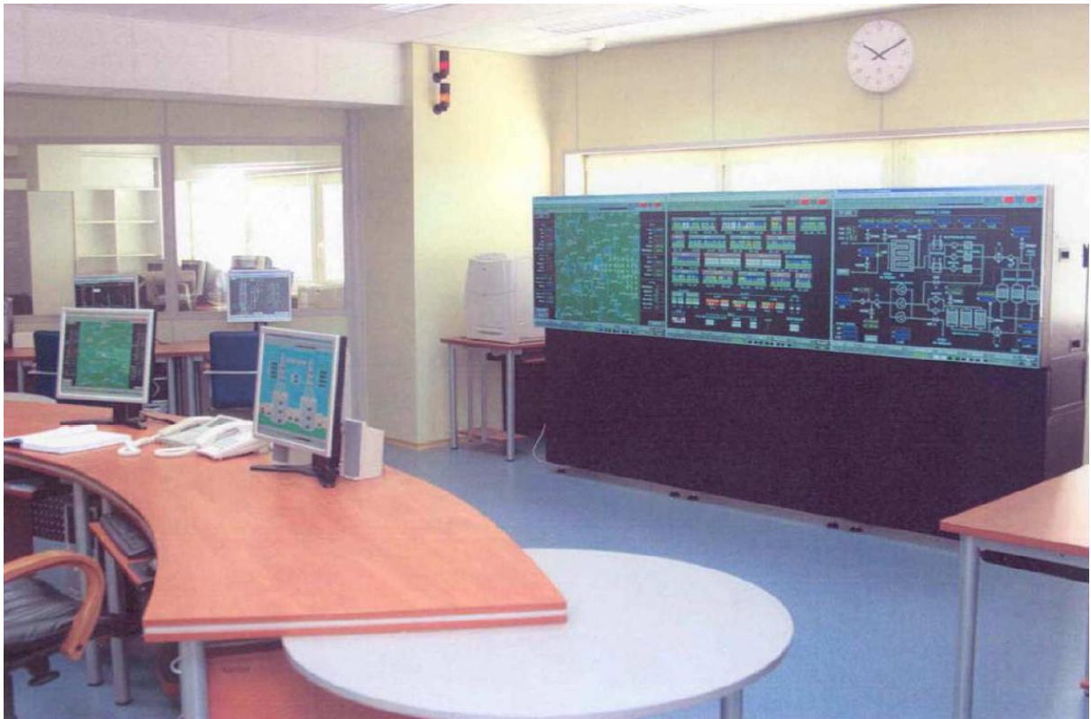
Figure 6.1-4. Radiation safety monitoring room with the automated radiation monitoring system
