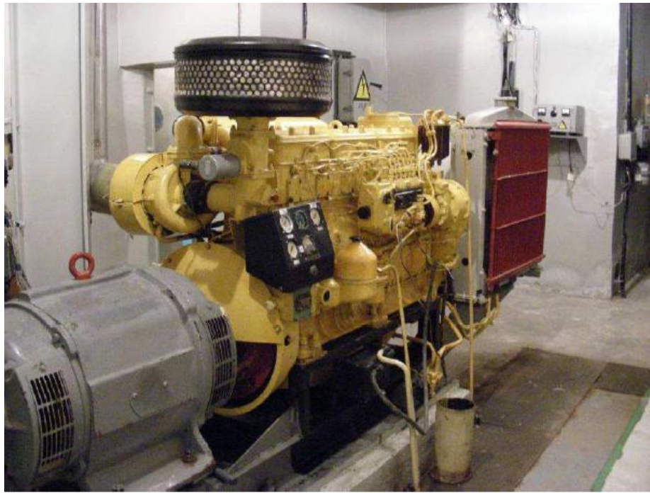
Figure 6.1-6. Stationary emergency diesel generator providing the OEP Accident Management Centre with power supply during NPP blackout
