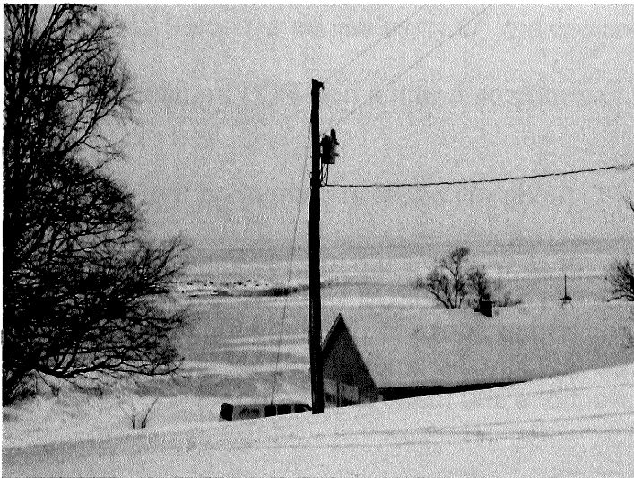
Figure 2. Example of a suspect transformer near Lake Superior.
