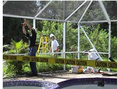
Warning tape for hazardous area
